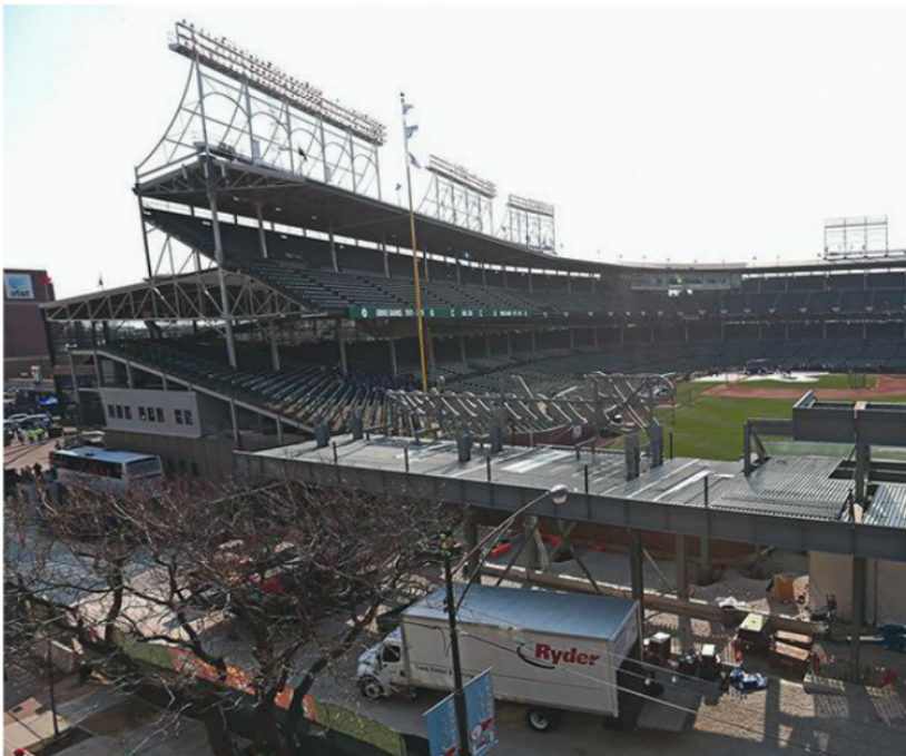
Service Wire's fast response helped Crescent Electric Supply meet a tight schedule that electrical contractor ABCO Electric faced during the Wrigley Field renovation.
